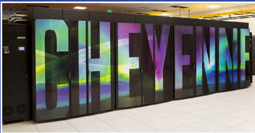
The Cheyenne supercomputer, which came online in 2017, is operated by the National Center for Atmospheric Research (NCAR). Housed in the NCAR-Wyoming Supercomputing Center, Cheyenne is one of the world's most powerful and energy-efficient supercomputers, with a theoretical performance of more than 34 million calculations per second for every watt of power consumed.
